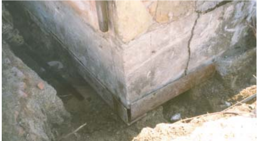
Above, angle iron is in place under an Amherst, N.Y., residential footing at the start of a helical pier foundation jacking job. Subsidence of plastic clay subsoils has damaged an uncertain number of Amherst homes that were built on unreinforced concrete basements, but a state panel has shot down the town's move to mandate rebar in all basement walls.
